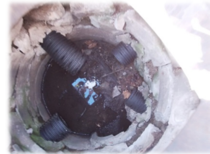
Wall Section Failure
