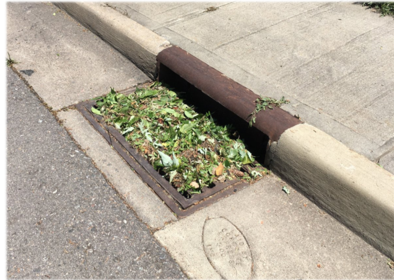
Figure: Clogged Inlet
