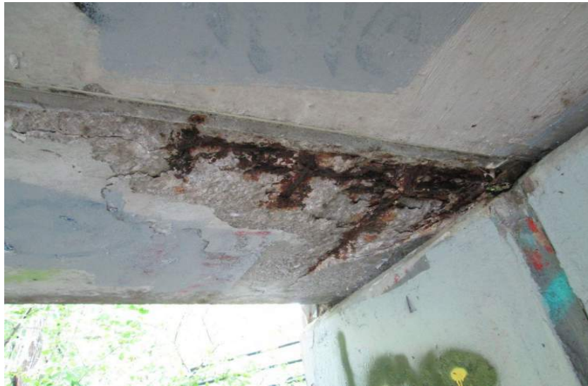
Stringers - East Span with Deterioration
