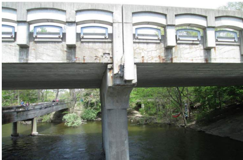
Fascia with spalling and cracking of beams at pier
