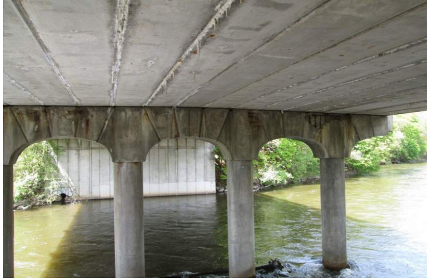
Pier West with Spalling
