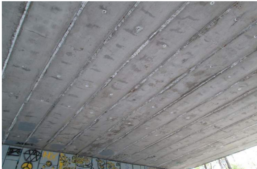
Stringers - East Span – Efflorescence between box beams and many longitudinal cracks in beams
