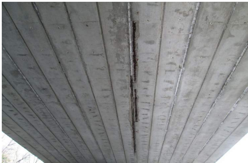
Stringers West Span– Efflorescence between box beams and cracking with exposed rebar
