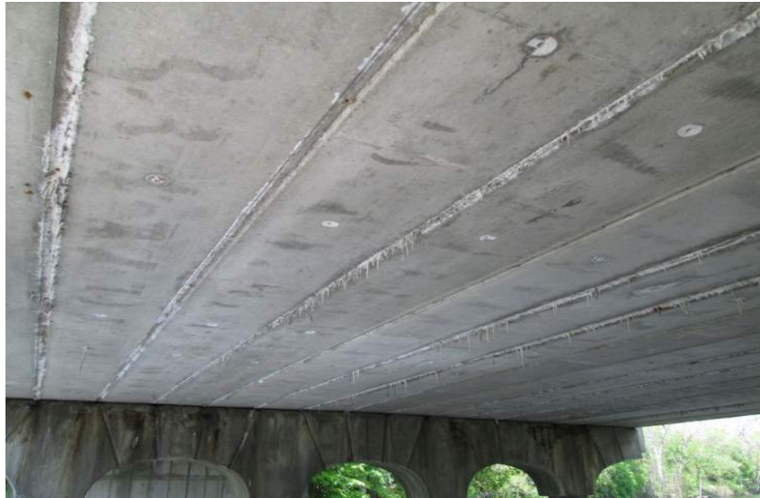
Stringers Middle Span– Efflorescence between box beams and many longitudinal cracks in beams
