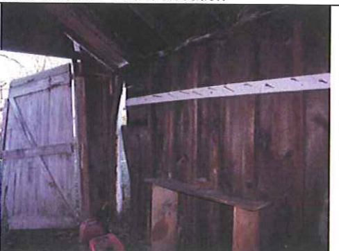
Shed interior – northwest corner; broken door, no frame, damaged corner, replacement sheathing.
