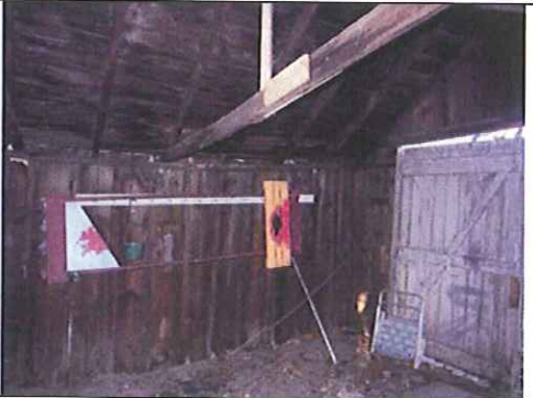
Shed interior – southwest corner; sagging eave, rotted bottom of siding boards, dirt floor, no foundation, not anchored to the ground.
