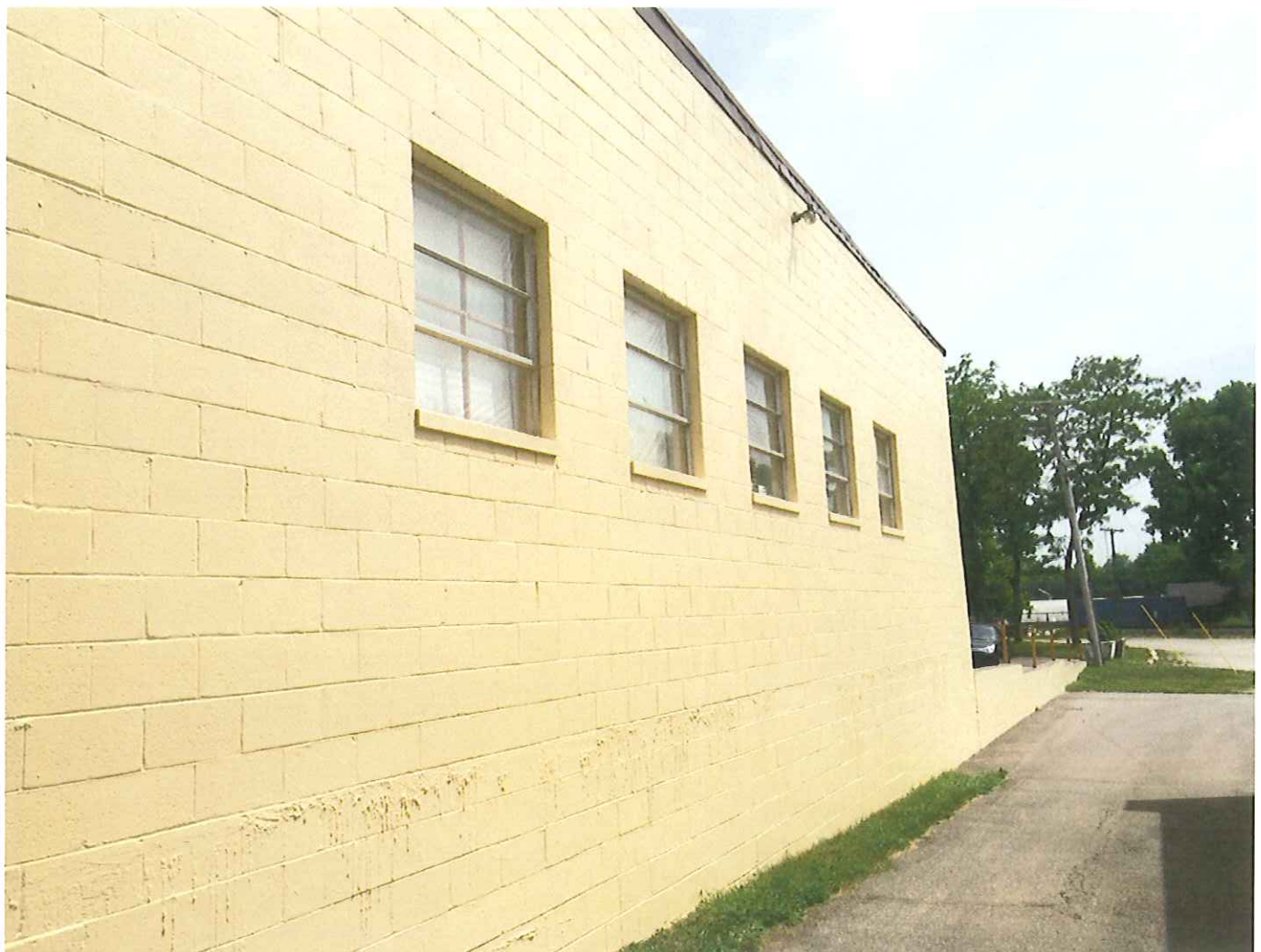
West side of Building - 5 windows to be replaced
