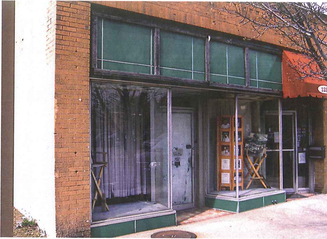
Current look of front facing. Window display on right side is destroyed and boarded up.
