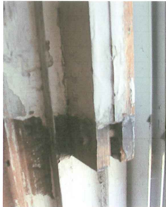
Photo 4. Broken window with stile remaining in jamb. Lower section of stile shows a wooden pin running through the mortise joint.
