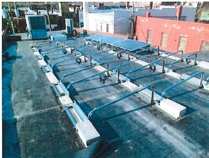
Setting up the racking
