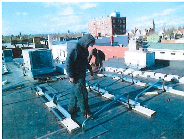
Final solar installation from above
