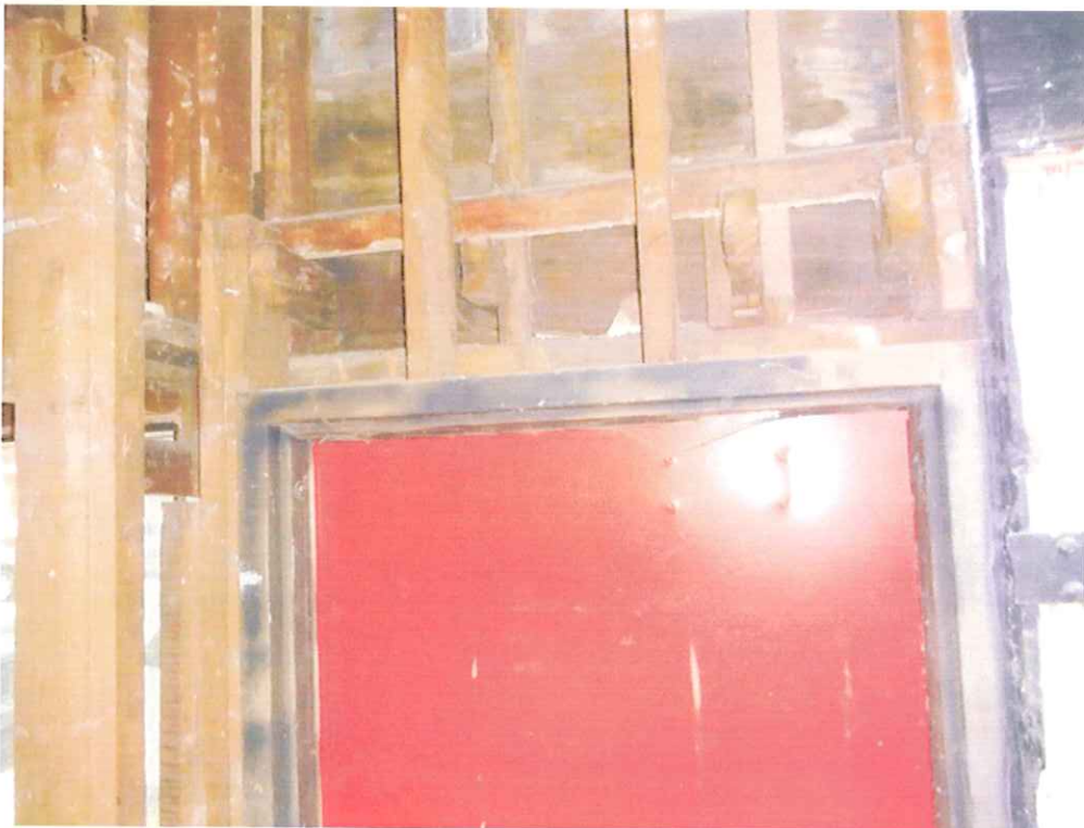
Photo #8 - At south door – the back-span of 2x4 canopy rafters has either been cut off and interior soffit removed or else never existed and an exterior suspender was always required.
