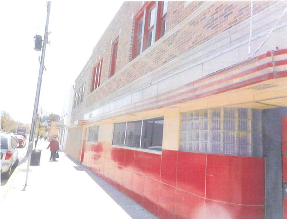
Photo #3 - Looking southwest. Note sag of window head.
