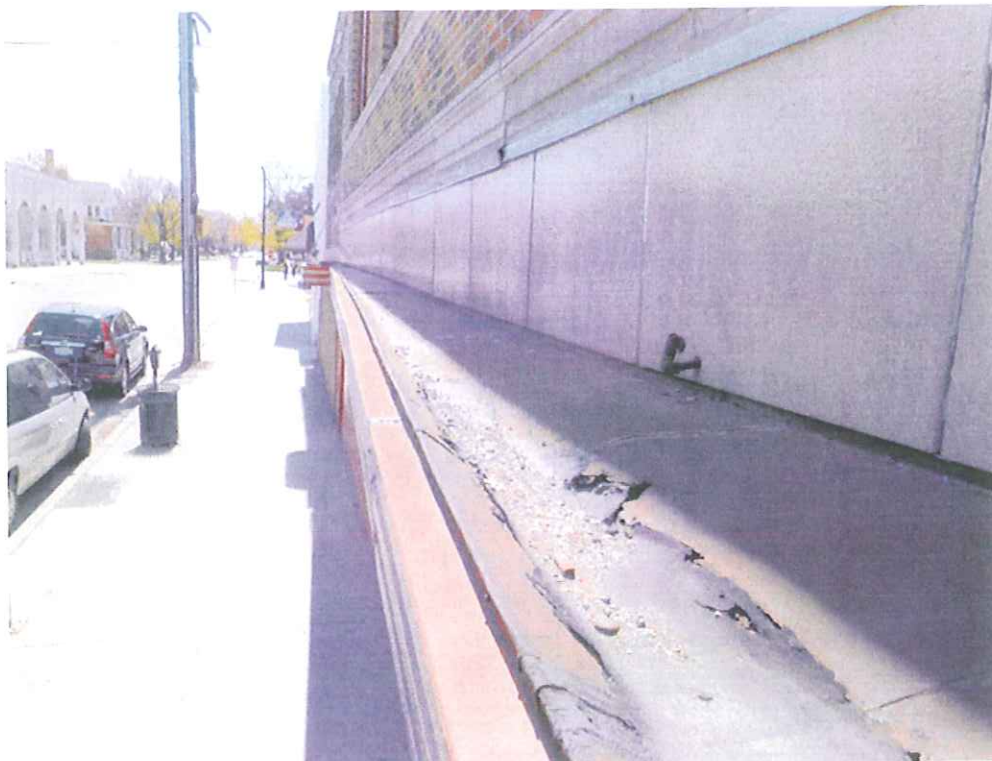
Photo #6 - Looking south. Note deteriorated condition of metal roof.
