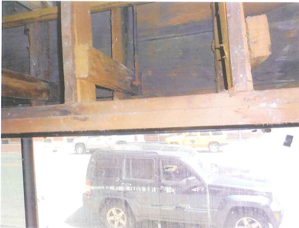
Photo #7 - Method of canopy support is via cantilevered 2x4's protruding through exterior board sheathing.
