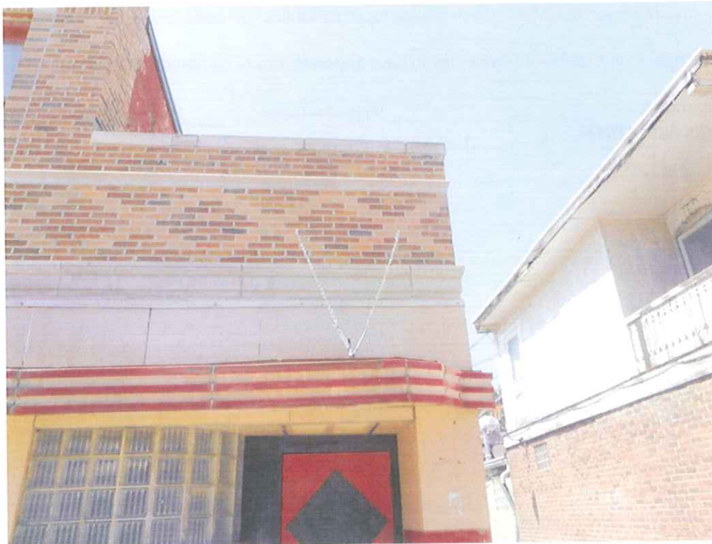
Photo #2 - Non-original chain and turnbuckle suspenders at north end.
