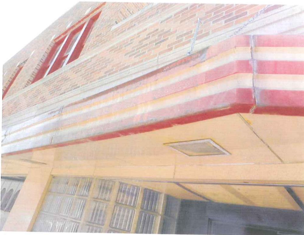
Photo #12 - Rusted condition of fascia near north end.
