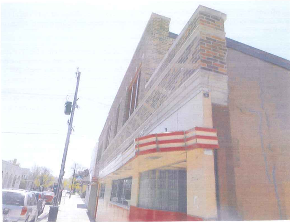
Photo #1 - Looking south. Note downspout at north end of canopy is the only drain.
