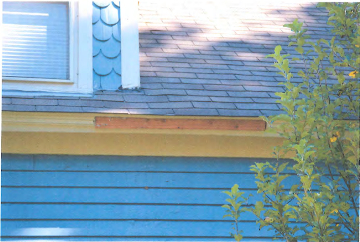
Up close view of dormer and damage
