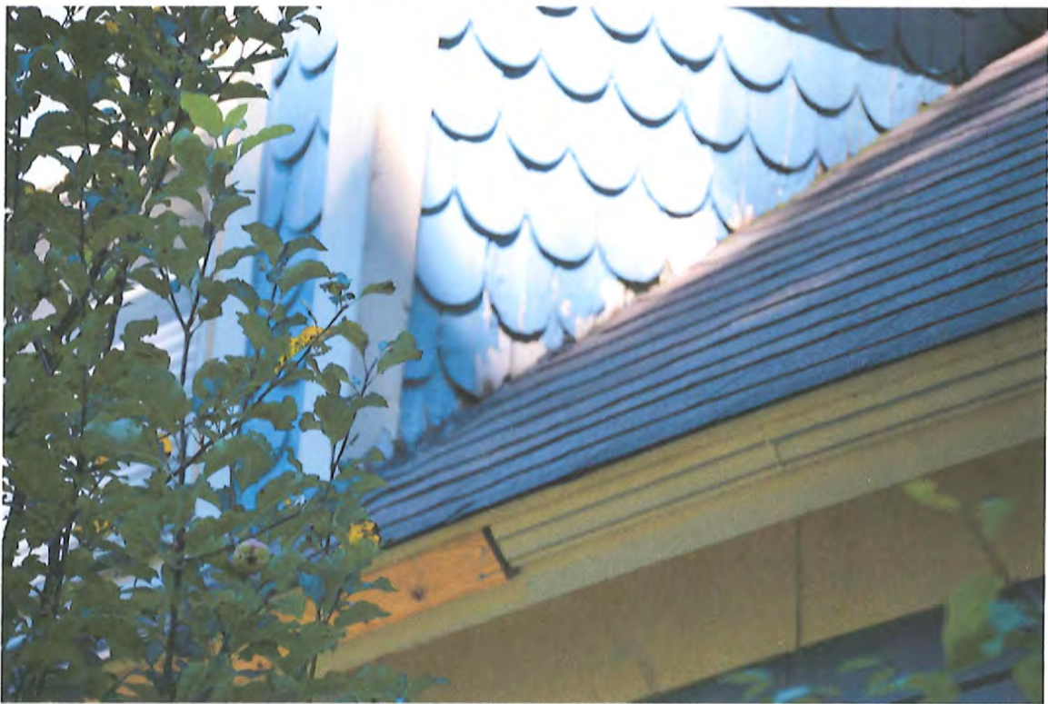
View of inadequate edge where dormer meets roofline.
