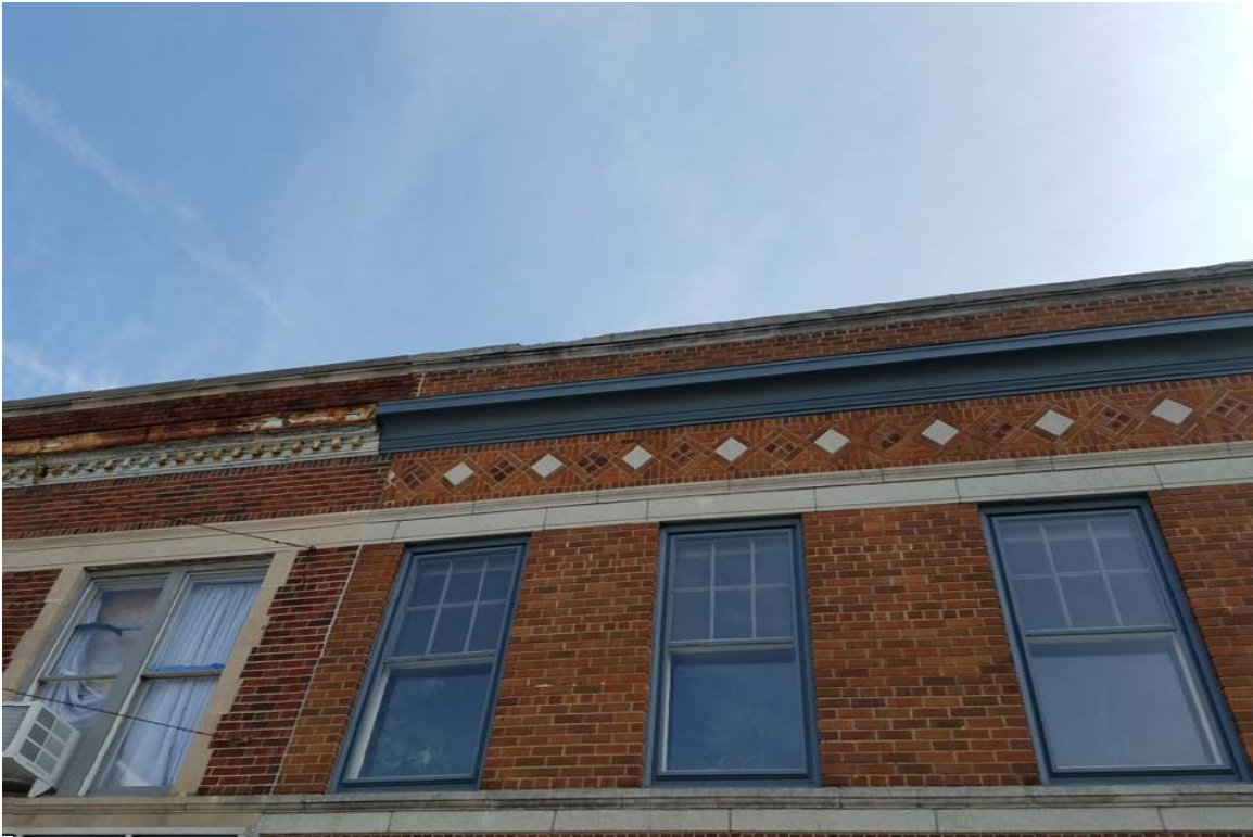
32-42 N Huron, facing east to facade parapet. Photo showing damage to the coping.
