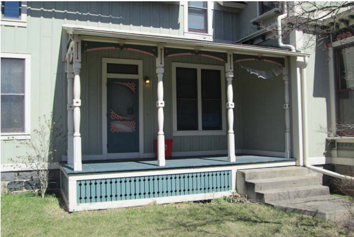
South elevation porch with deck to be replaced.
