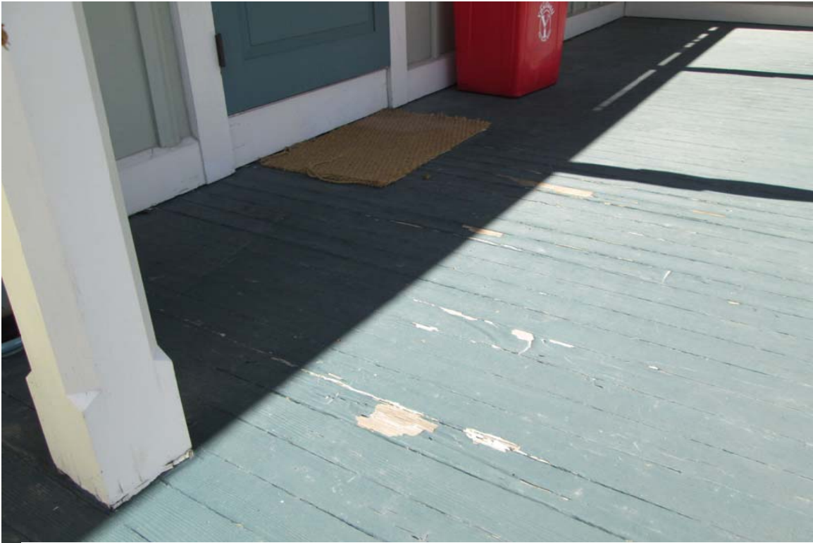
Photos showing deterioration and current conditions of porch deck
