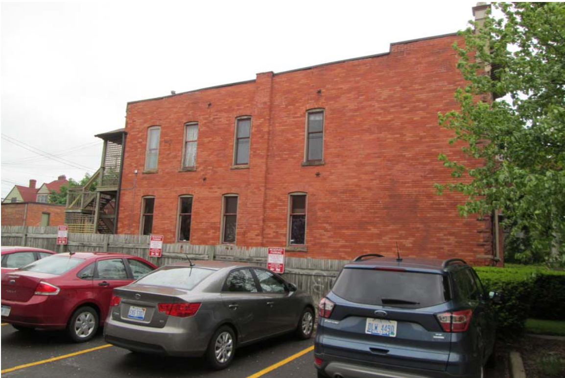
Facing northwest to south elevation. Windows to be repainted/repaired.
