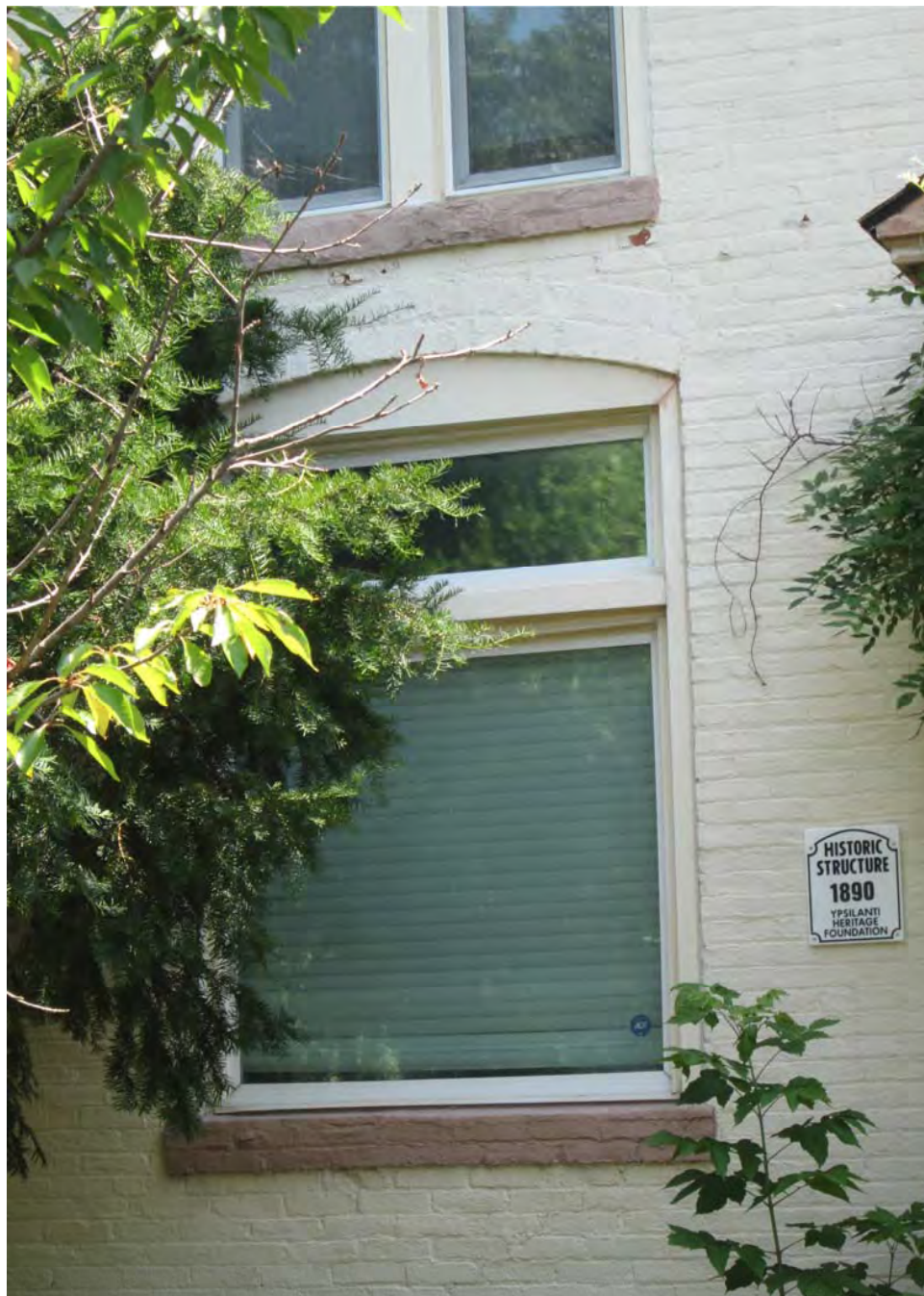
Staff photos: 216 N Grove, facing east to facade showing window to be replaced.
