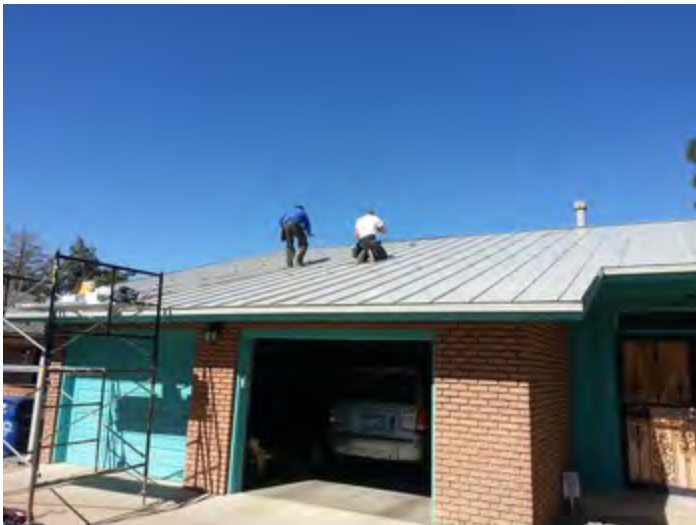
Mounts on Roof
