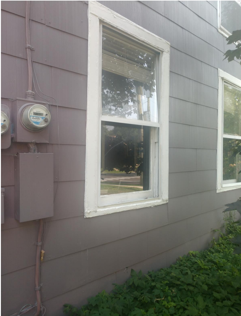
Window #2 Driveway side
