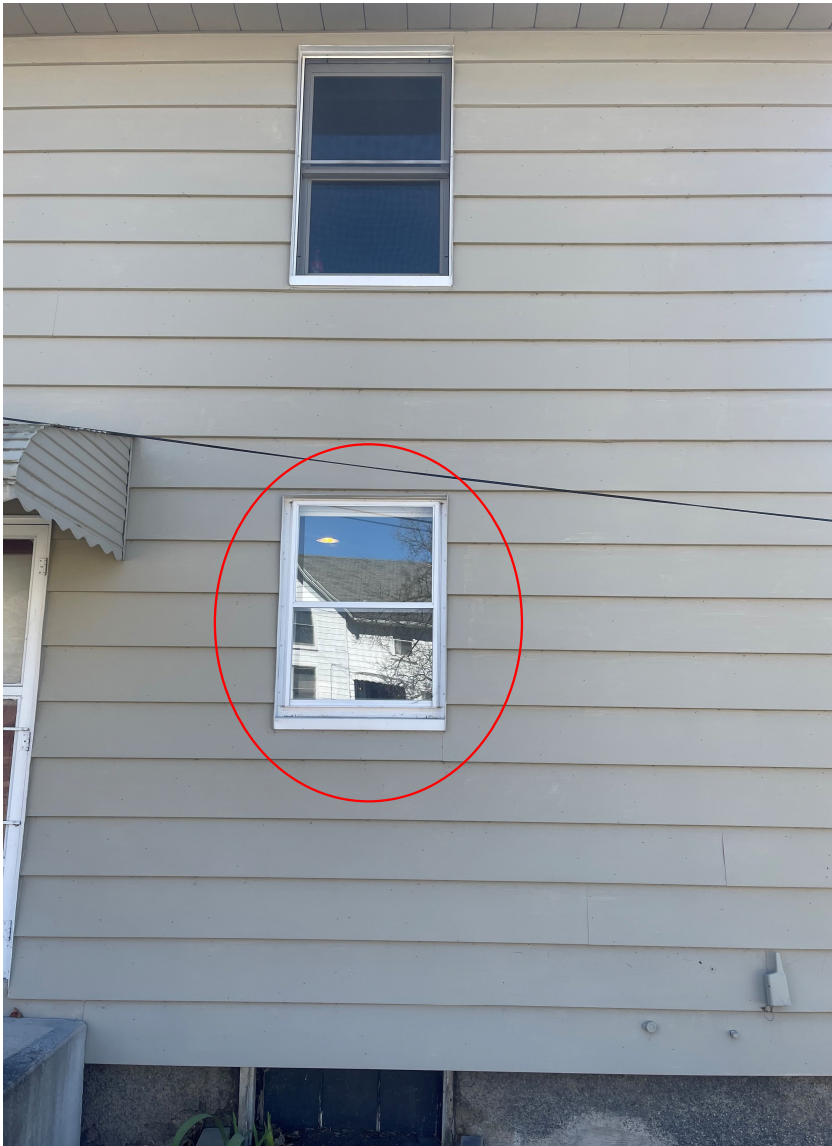
First story window on north elevation to be replaced.
