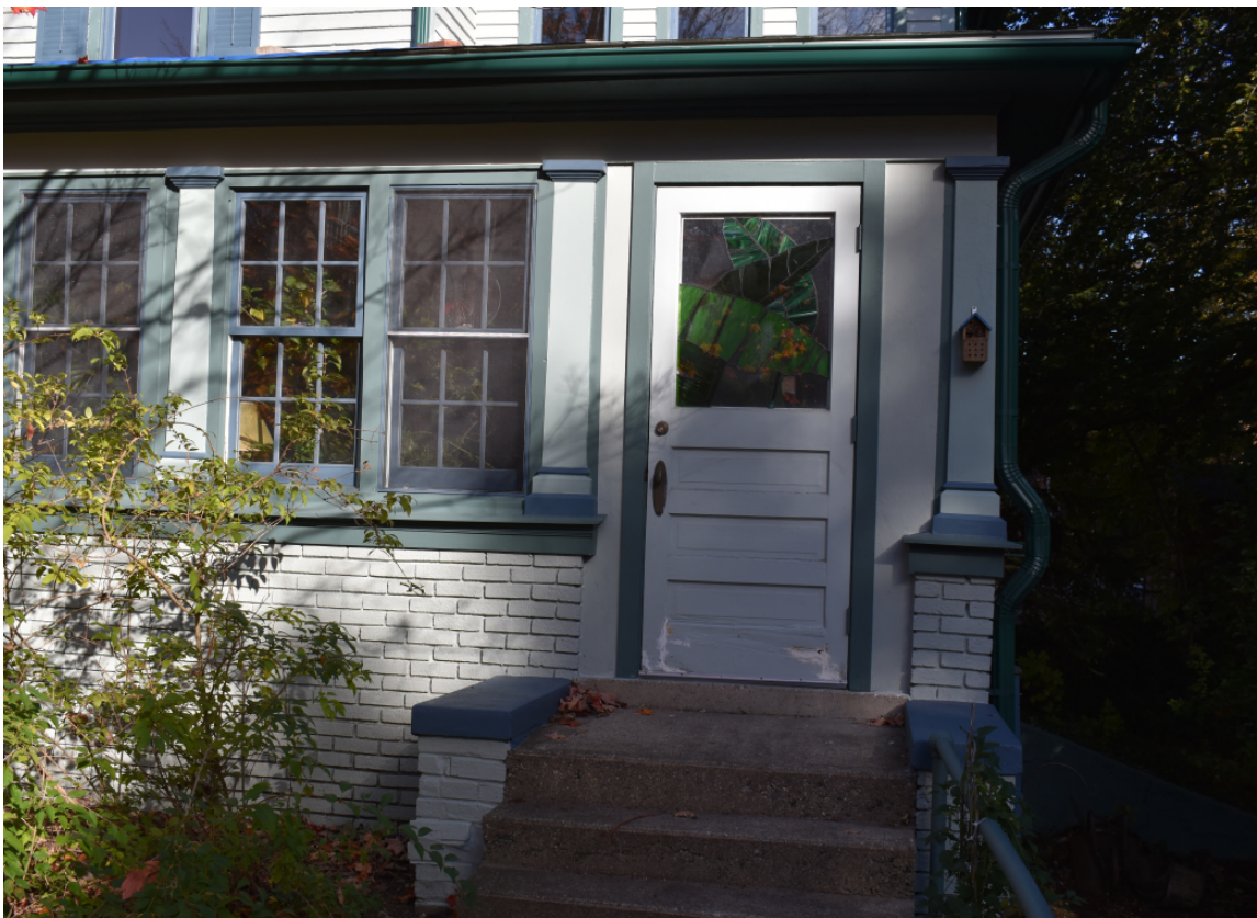
Facing north to south door that has been damaged by ants
