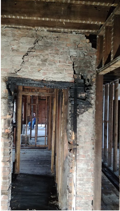
Figure 4: Failing Bearing Wall
