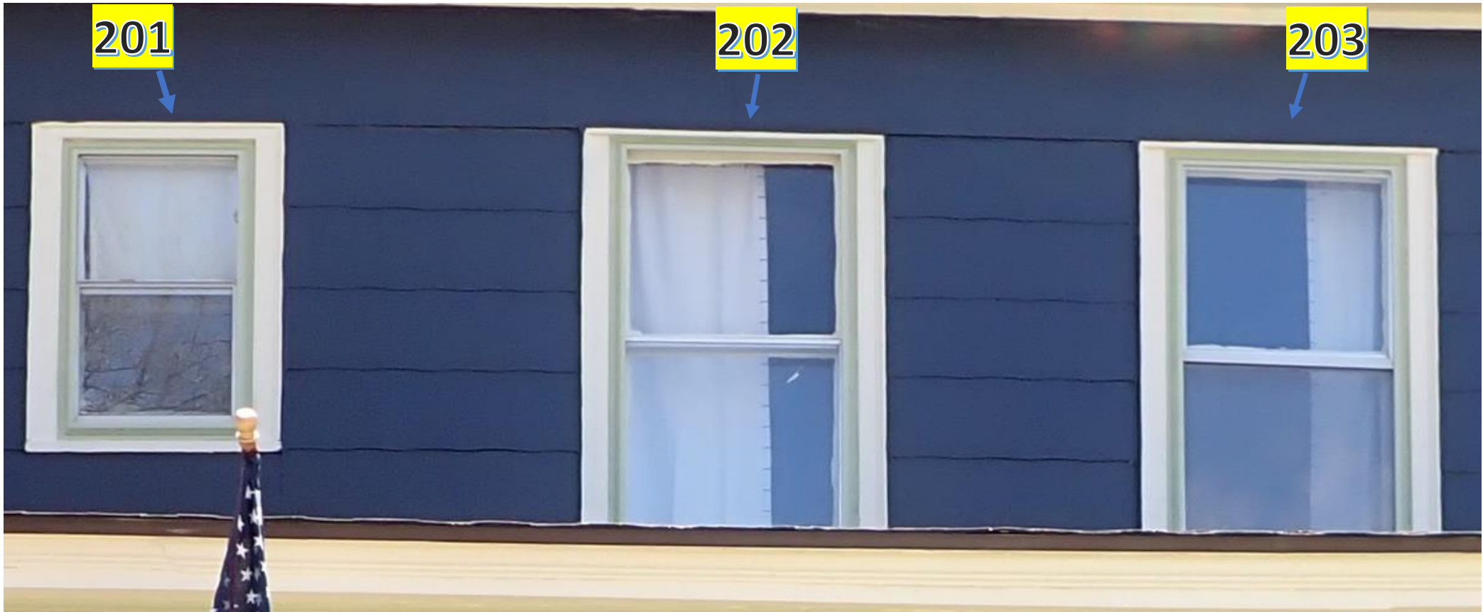
Front of house - 201 is framed differently on top compared to 202 and 203
