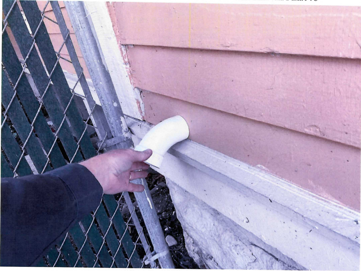
Washington, 315 S -Water heater vent. 2-inch PVC
