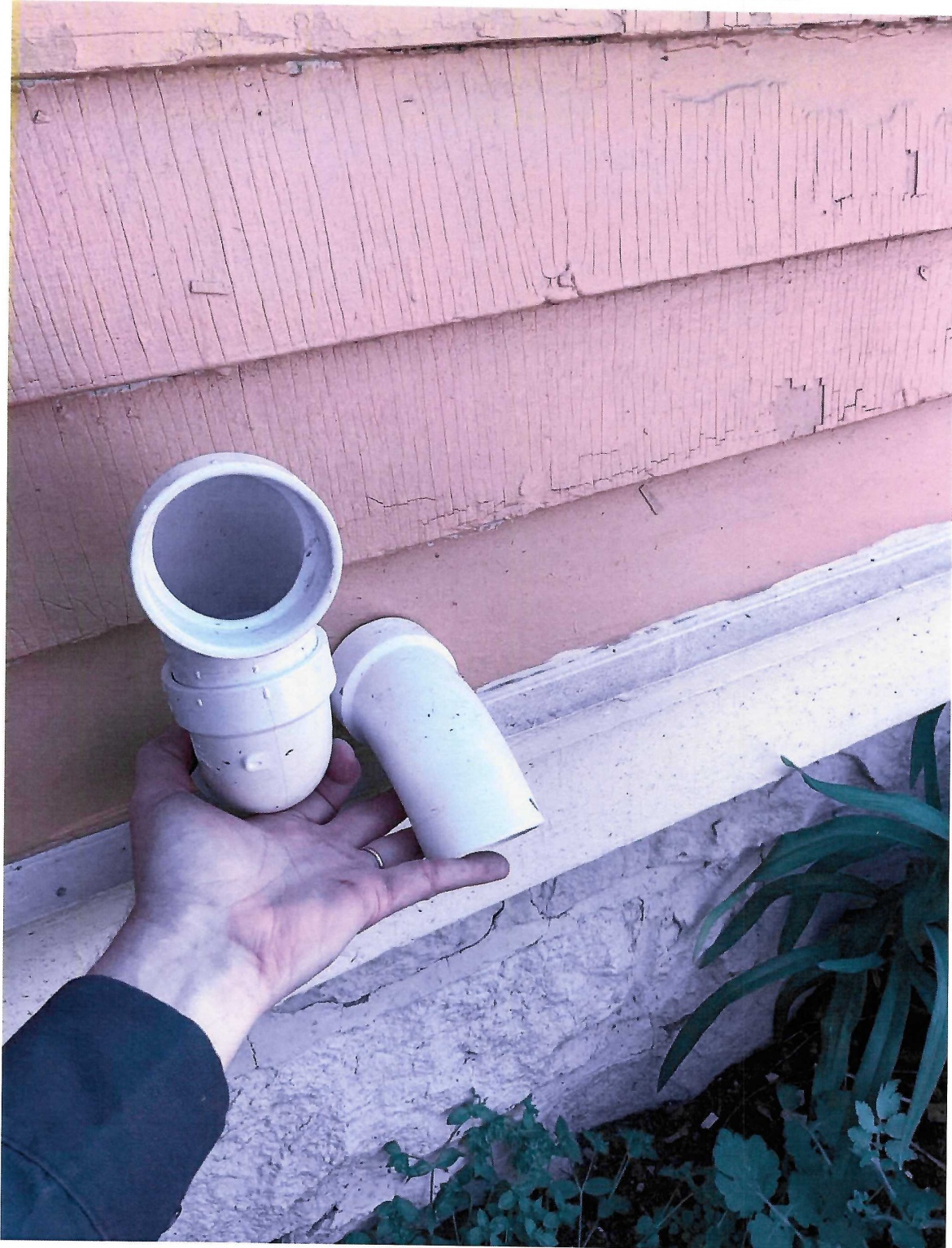
Washington, 315 S -Furnace vent
