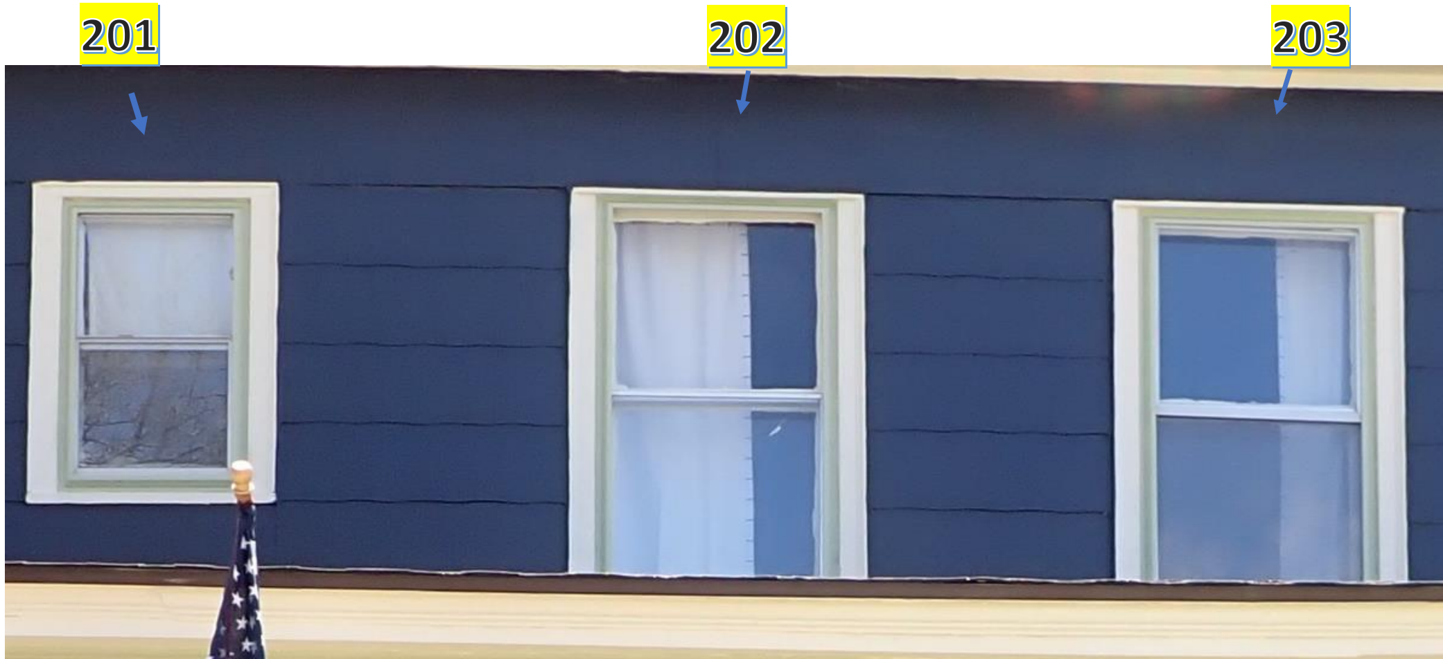
Front of house - 201 is framed differently on top compared to 202 and 203
