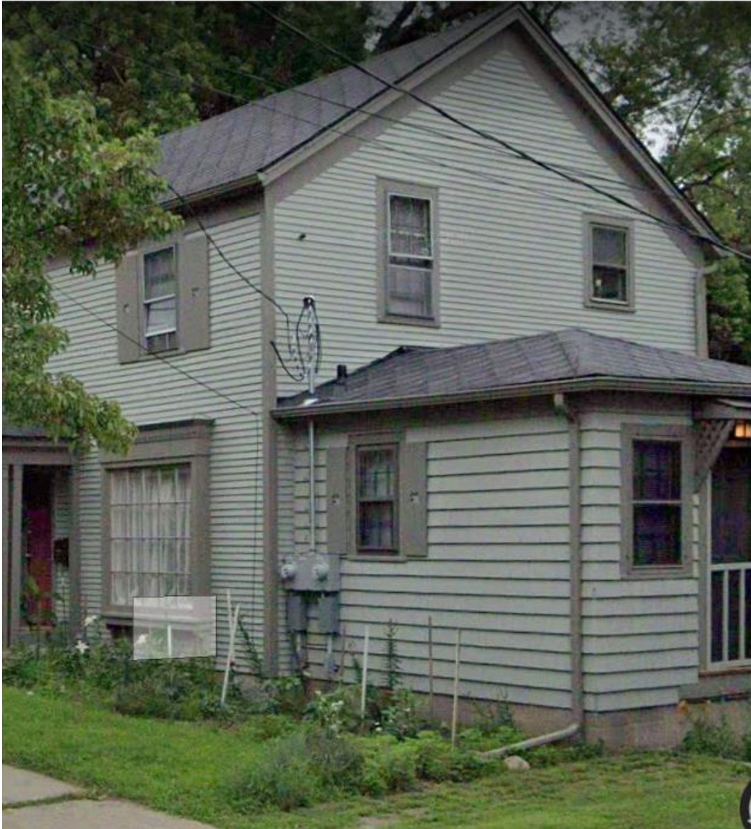
New meters and conduit visible (Google, July 2019)
