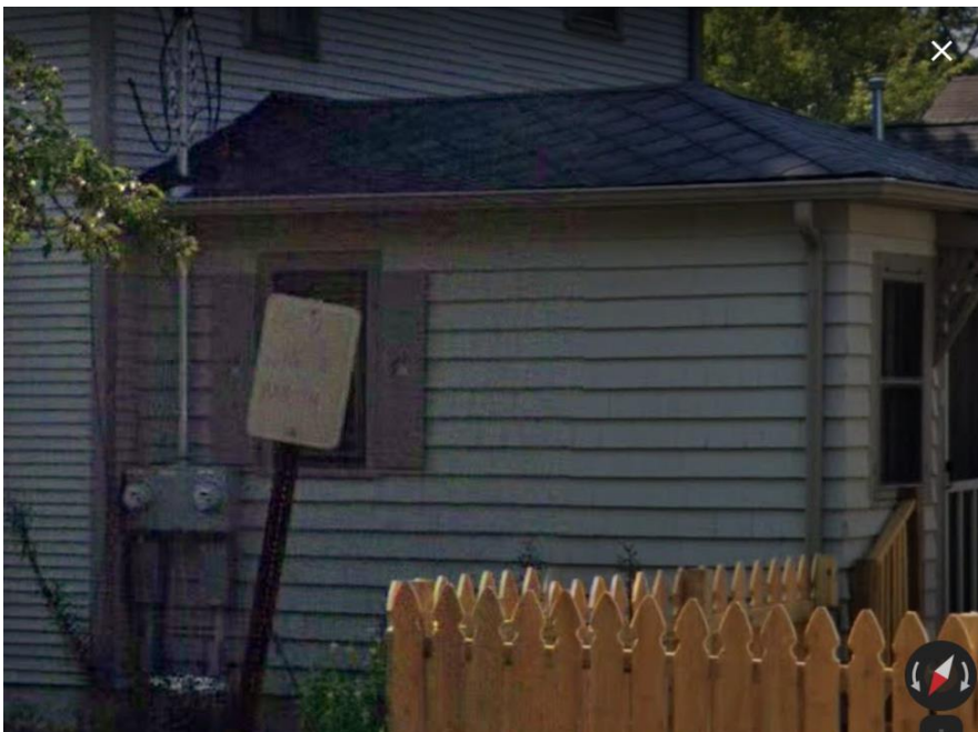
House, front (north) side, one-story addition detail showing meters and conduit. (Google, June 2021)
