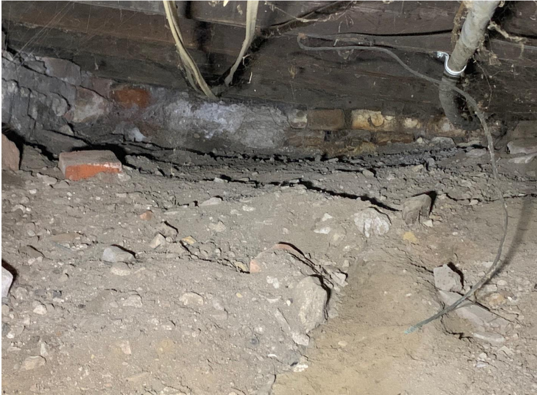
Kitchen Northwest Corner 2—the pile of dirt almost touches the joists above
