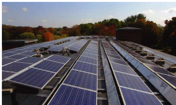
Solar panels installed on the flat roof.
