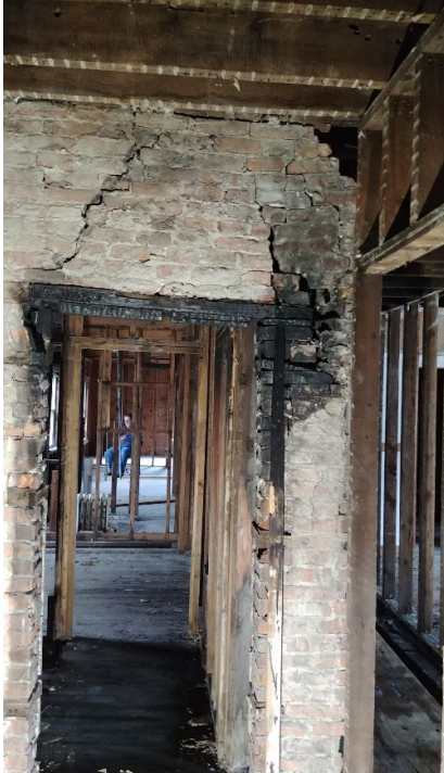
Figure 4: Failing Bearing Wall
