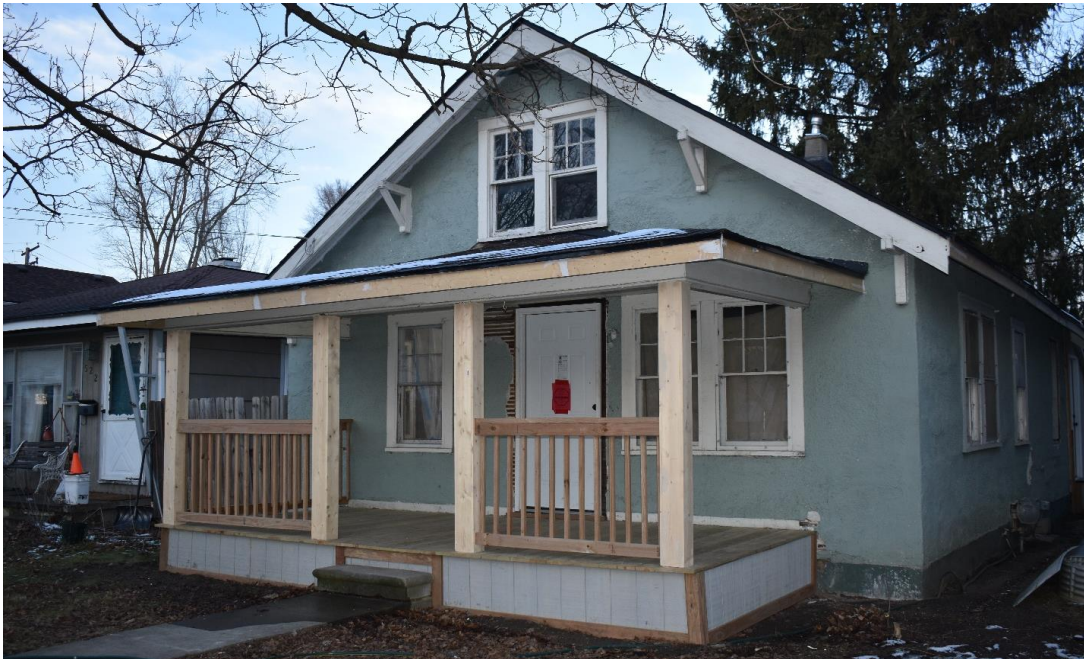
January 2023, staff photo of work that had been completed without permits.
