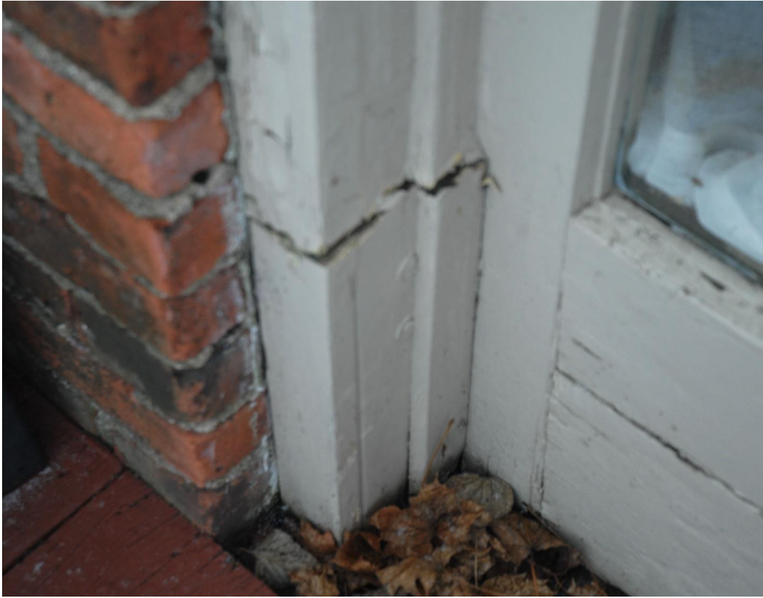
Evidence of wood trim pieced in after years of deterioration, likely caused by the negative grade.
