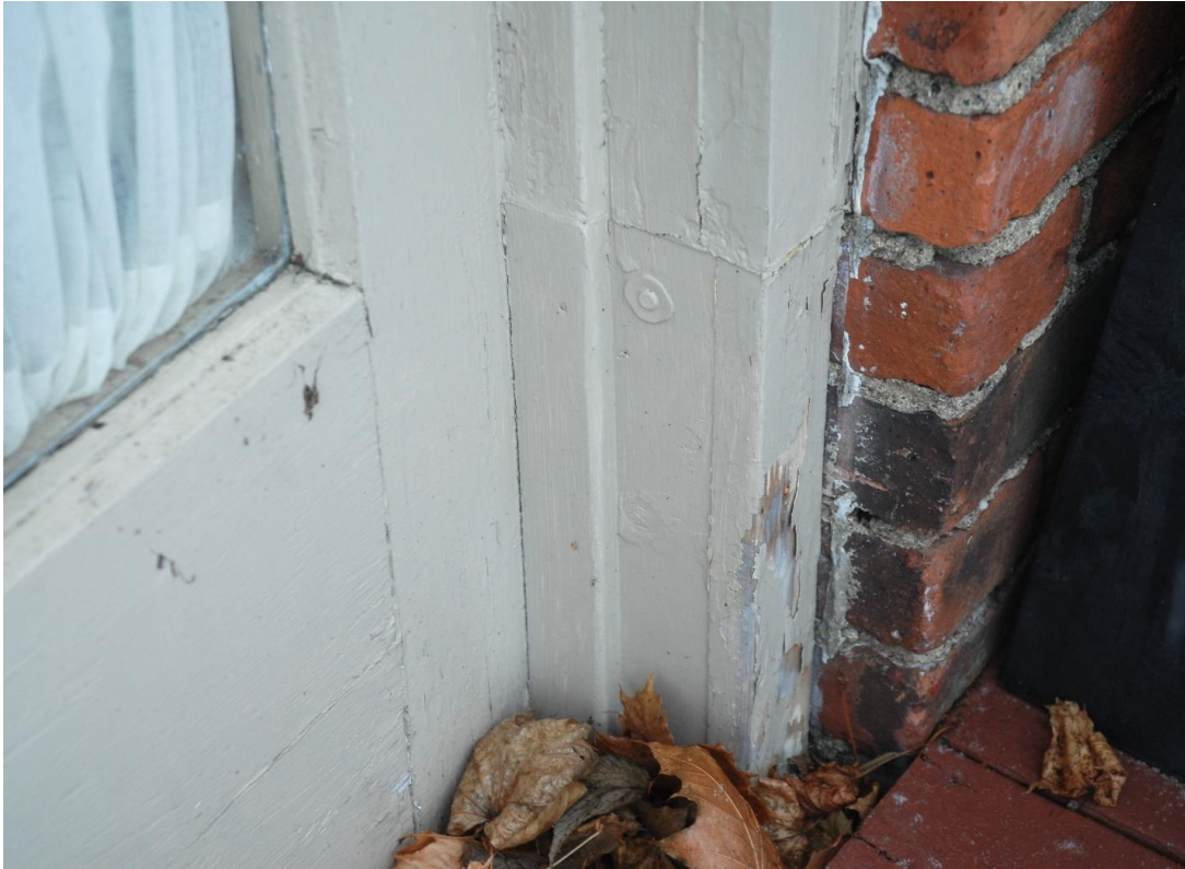
Evidence of wood trim pieced in after years of deterioration, likely caused by the negative grade.
