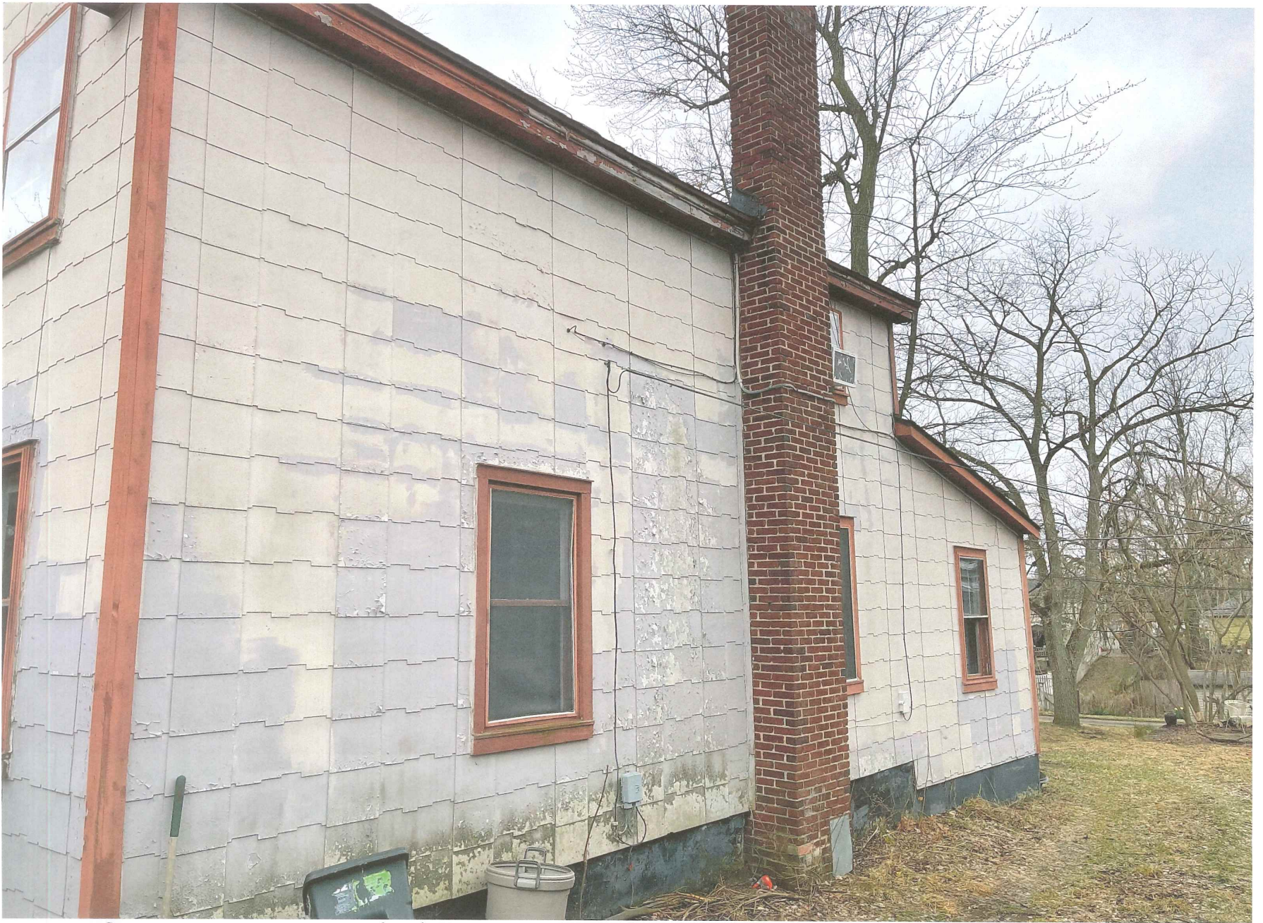
627 N River, north side. Siding proposed to be removed & wood siding underneath repaired.
