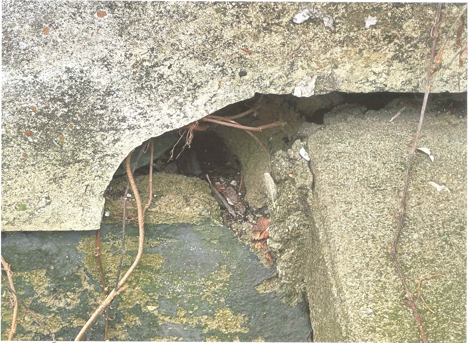
DETAIL of Front (EAST) side of house, recessed porch area showing separation of concrete & siding. April 2023
