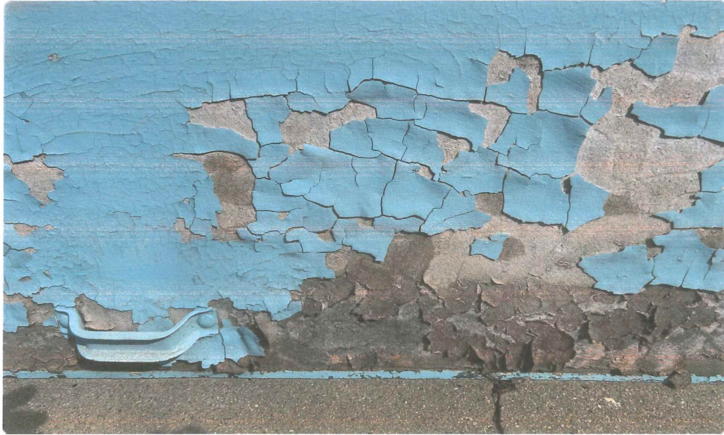
Detail of Particle Board Deterioration of Ex. Door
