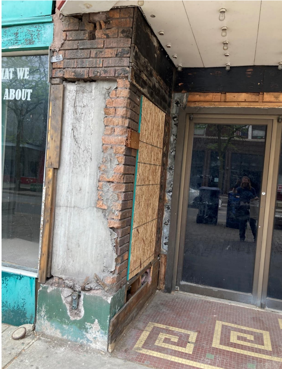
Figures 2- 7, below. Photos showing damage from removing the gravel veneer that had been applied to the walls of the alcove under the marquee.
