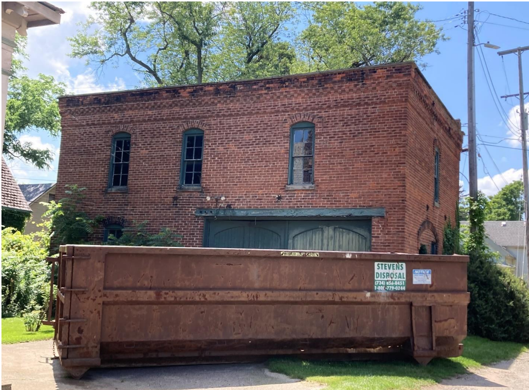
Fig. 6. Italianate carriage house, also contributing to the district. Conditions assessment noted that it has open flashing and eroded roof coating. Unclear to staff if the carriage house will get an EPDM roof or perhaps some other option.
