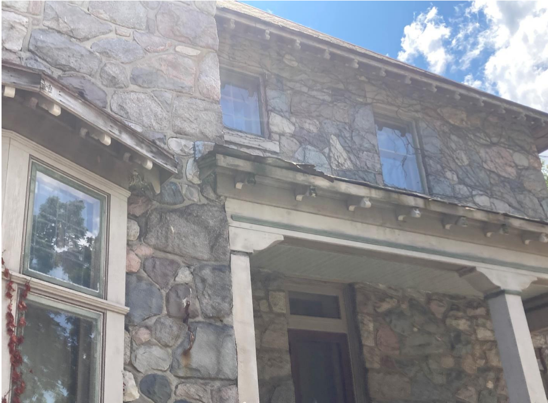
Fig. 5. 212 S Huron, north side porch detail of roof damage.
