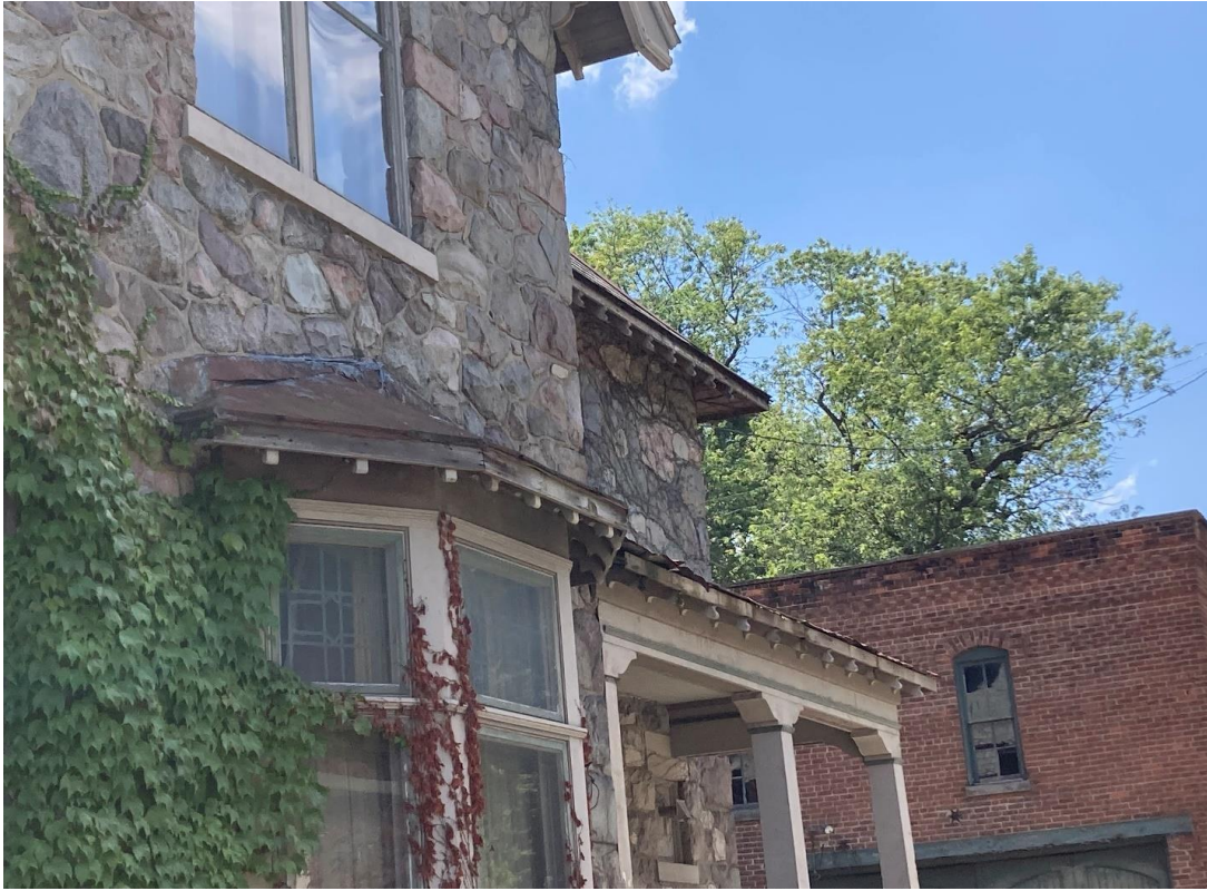
Fig 4. More detailed photo of north side porch roof and bay window roof, both deteriorated metal. Carriage house in background.
