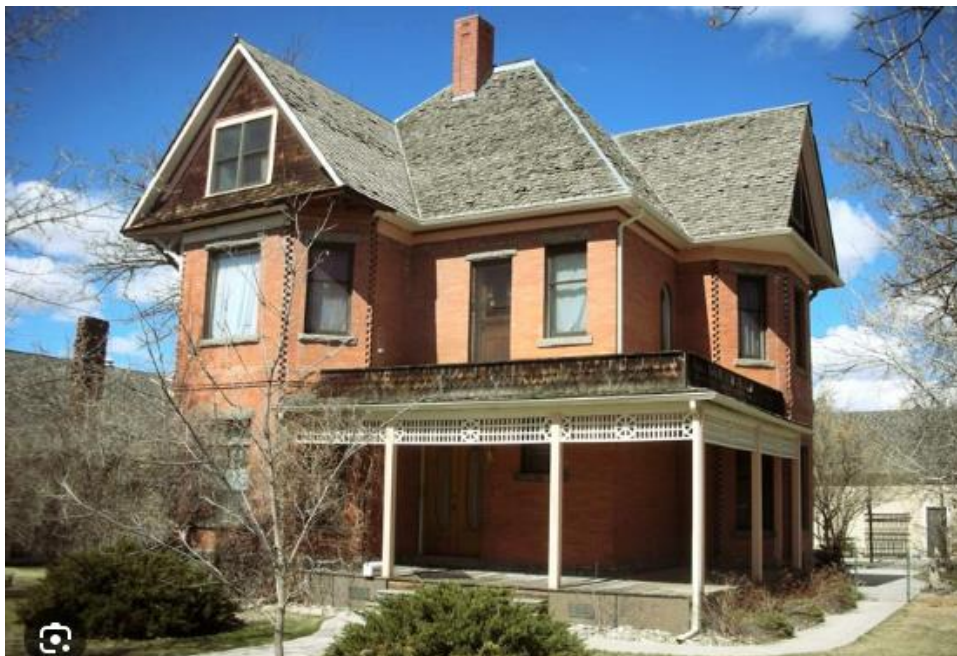
Figure 9. Photo from the image search as above. Queen Anne with an old shingle roof. Roof is in poor condition but the texture shingles provide complements the house's Queen Anne details.
