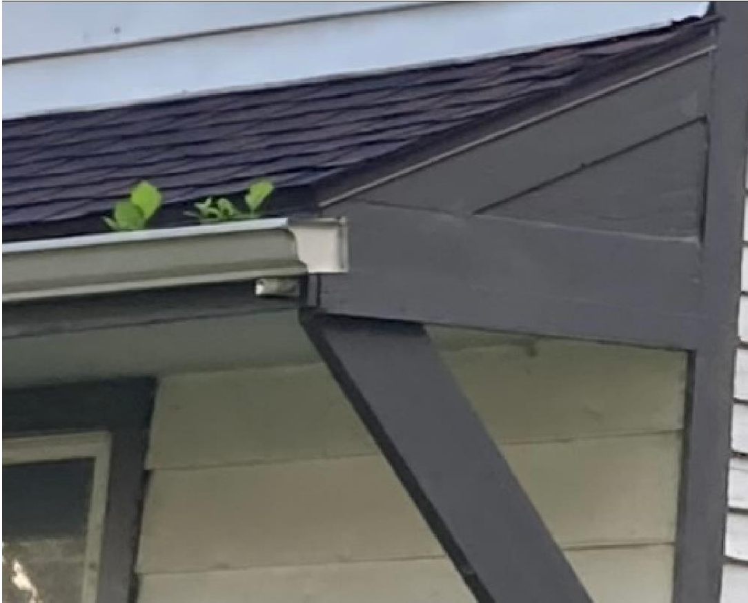
August 2023 staff detail photo of gutter, downspout stub, and wood porch roof support at 307 N Hamilton. Having the downspout hang straight down without attaching it to the house for support seems to staff like that will likely not function well or be in compliance with the design guidelines.
