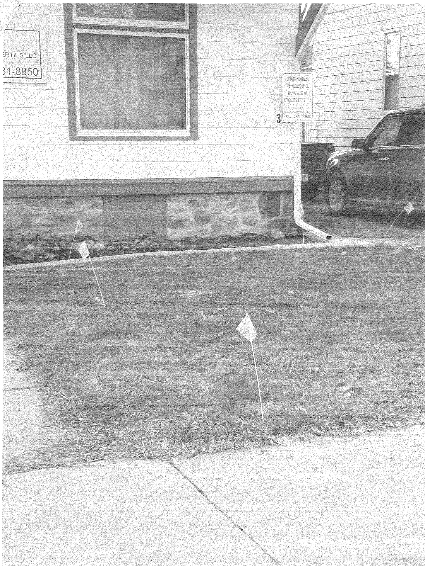
Photo shows how downspout follows the line of the bracket and then straightens out against the house at the NE corner. 8/22/23 https://mail.google.com/mail/u/0/#inbox?projector=1
