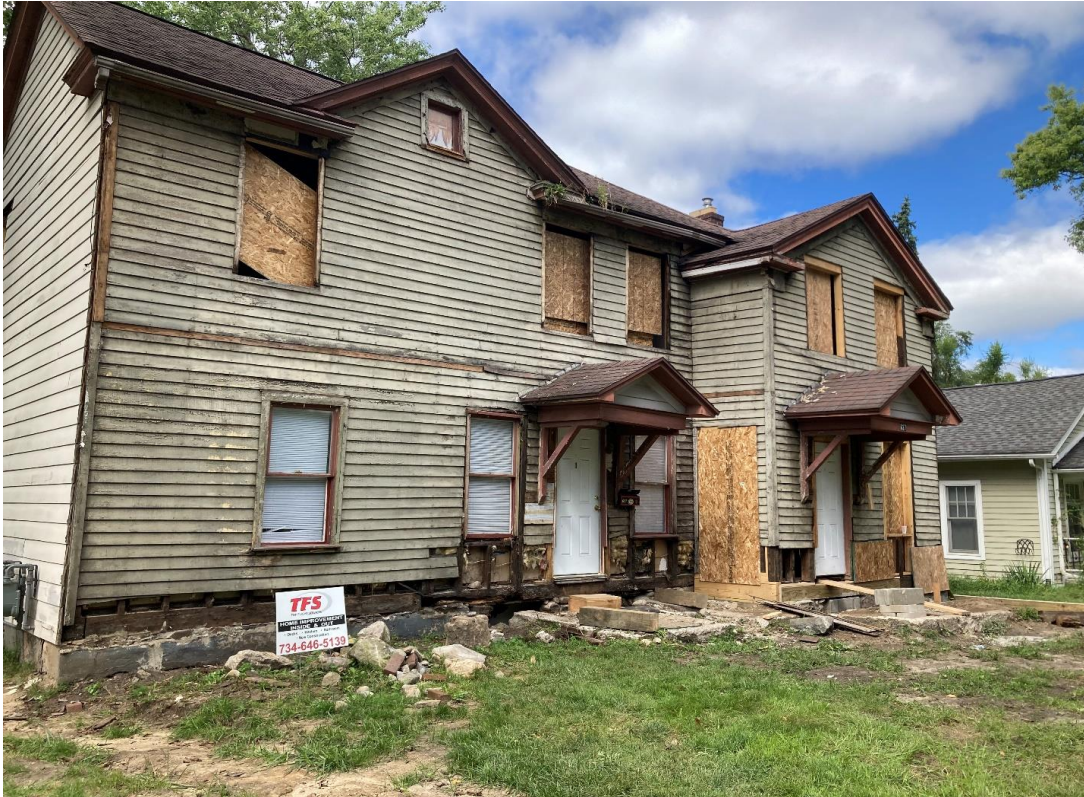
627 N River, September 2023. Staff suggests that the reveal of the lap siding on the front (east) side should be the benchmark for the siding reveal all the way around the house. The historic trim and cornice returns in the gable should be preserved and the new siding should look just like this siding where it interacts with that historic trim.
