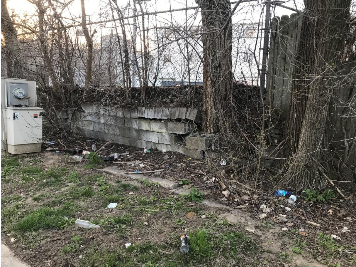
Figure 8: Crumbling block retaining wall (April 2020)
