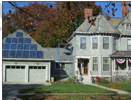
Figure 3. Solar array installed on Historic property in City of Ypsilanti.
