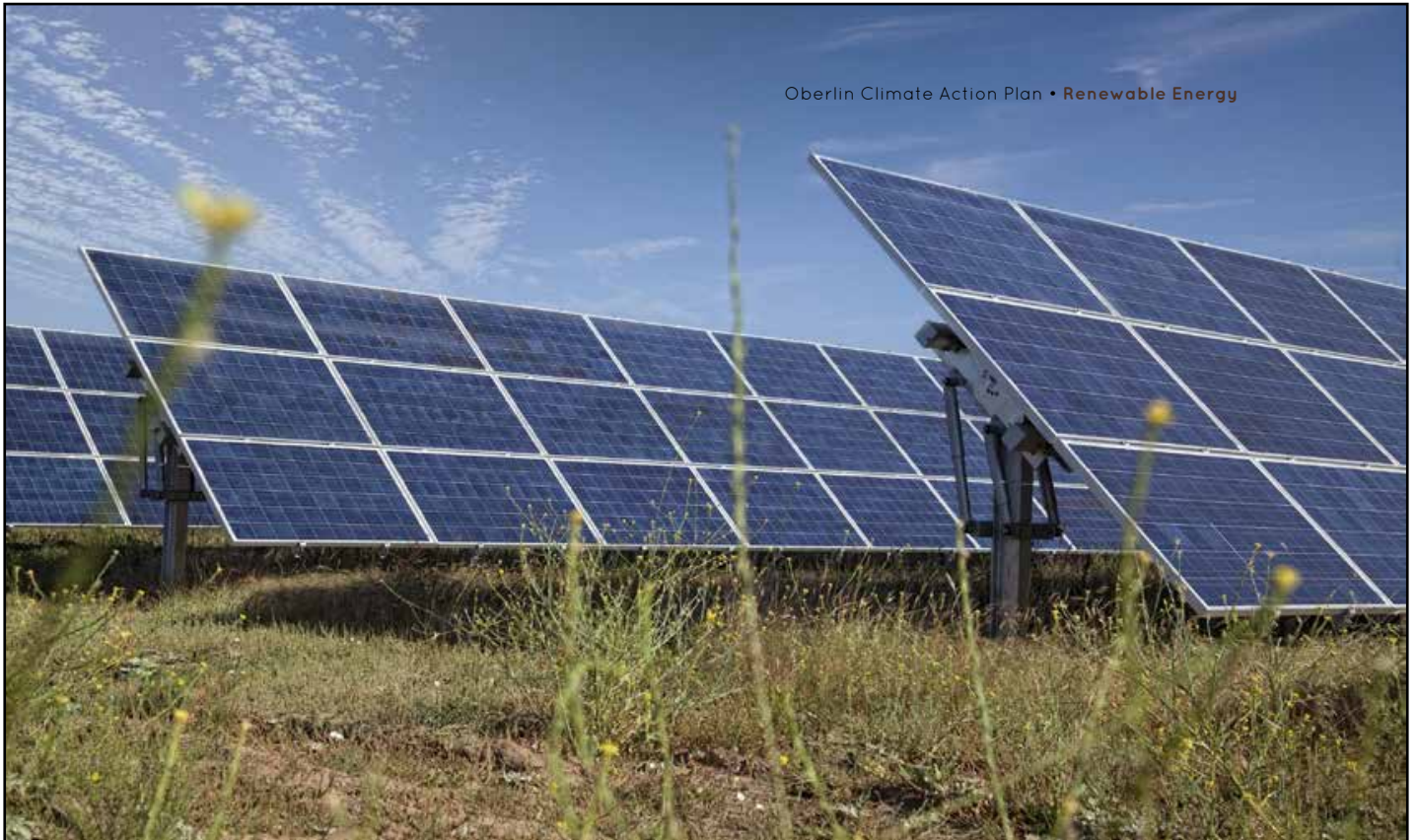
Rendition of the 2.27 MW solar array constructed on Oberlin College property in 2012. Photo by Rob Lamma for Oberlin College.
