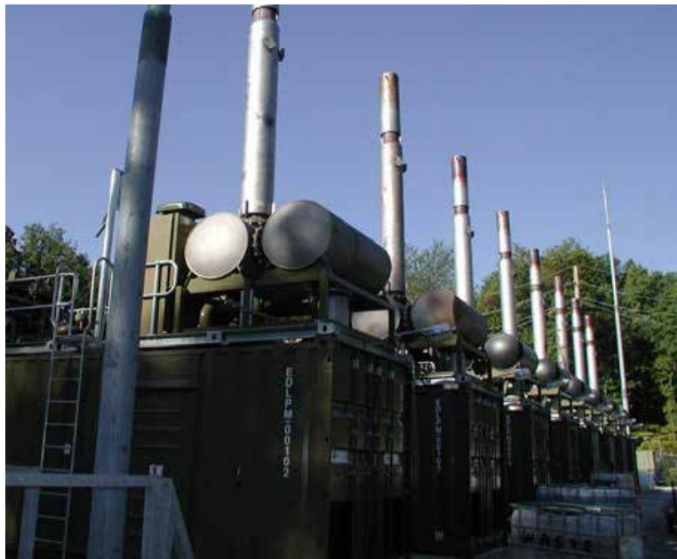
Landfill gas to energy generators at the Lorain County Landfill.
