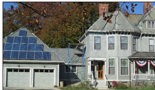
Figure 4. Solar array installed on historic property in City of Ypsilanti. Source: City of Ypsilanti.
