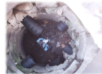
Wall Section Failure
