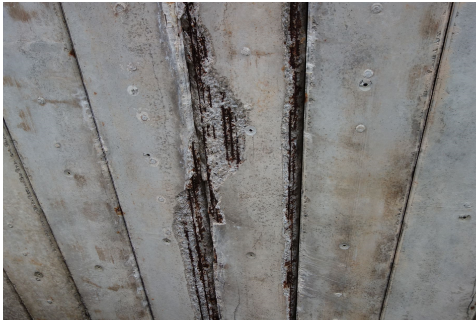
Exposed strands in beams
