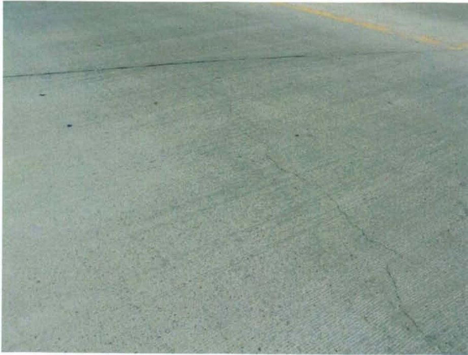
Surface with cracking
