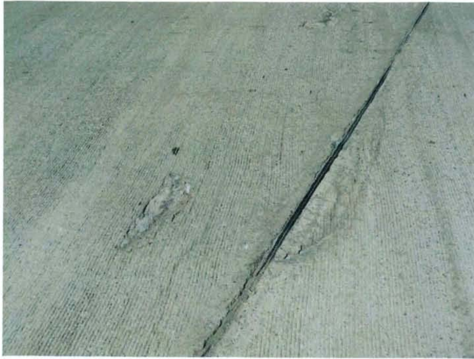
Spalling near the pier joint
