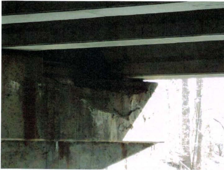
Pier deterioration in southwest quadrant
