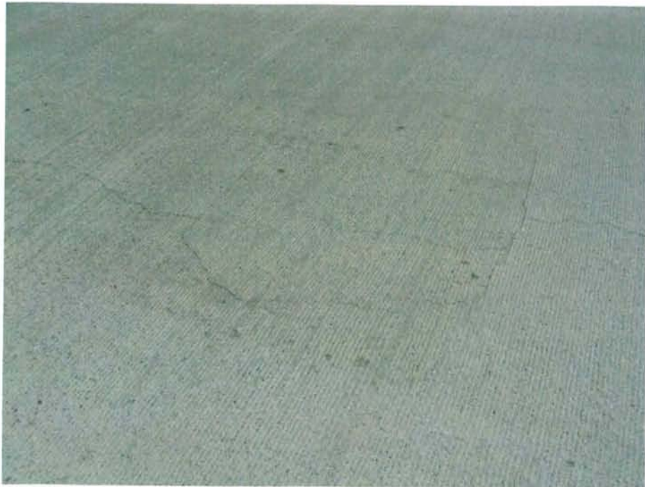
Surface with cracking
