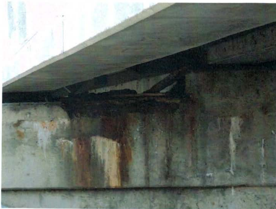
Pier deterioration in northwest quadrant
