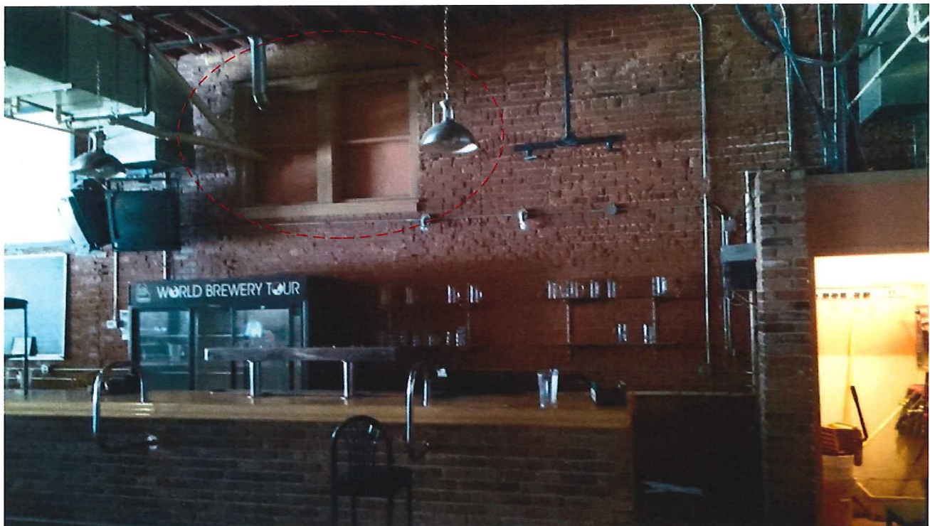
Interior View: note missing double-hung windows
