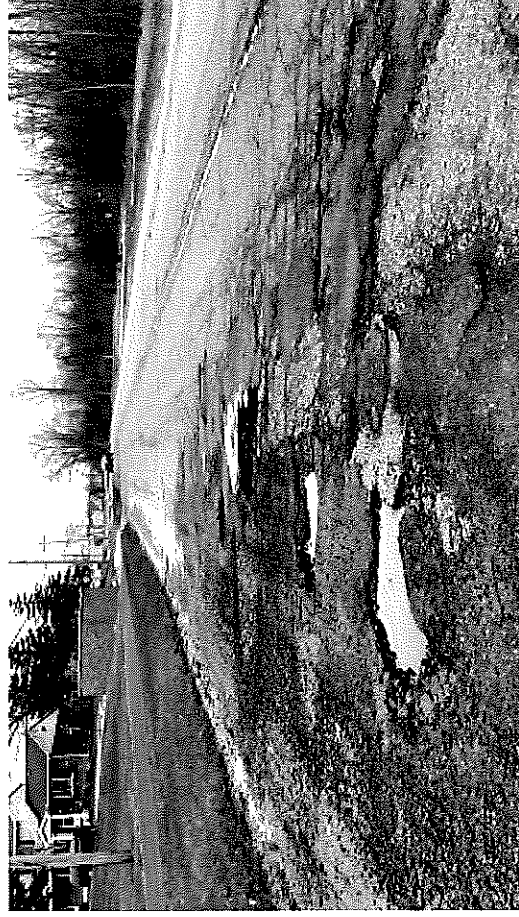
Current state of MacArthur Rd, would be improved in 2017 with 4-year millage
