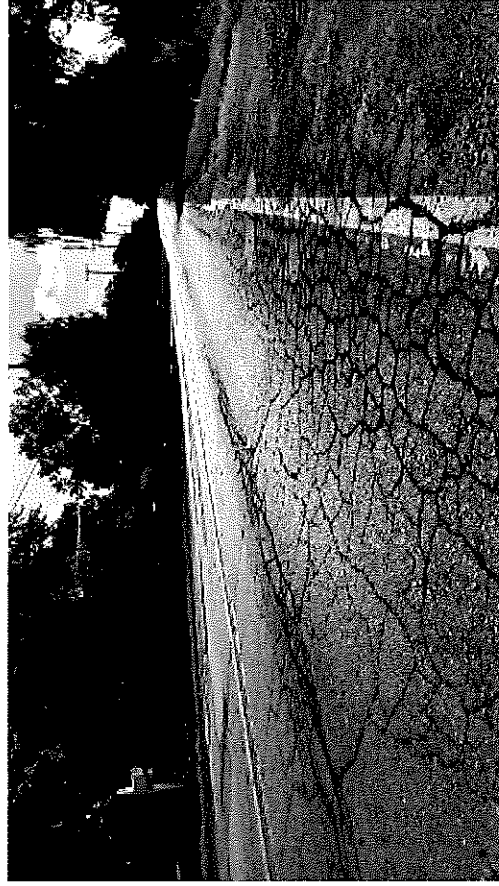
Current state of Six Mile Rd, funded by 2016 P.A. 283
