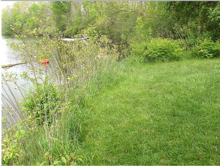
Photograph 1 – Upstream face of the left embankment viewed from the right Note the brush growing along the water line
