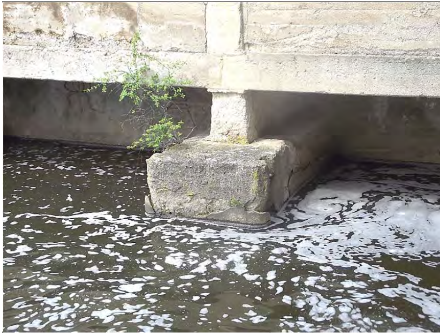
Photograph 25 – Close up of the deteriorated pier Note the vegetation
