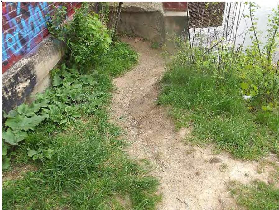
Photograph 2 – Foot traffic erosion at the upstream face of the left embankment
