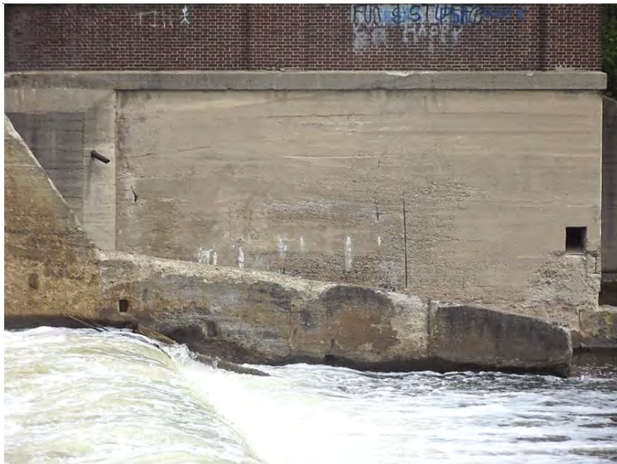
Photograph 16 – Downstream right principal spillway abutment wall Note the significant deterioration
