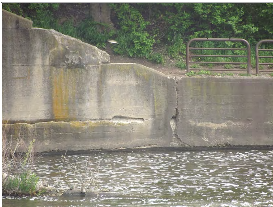
Photograph 27 – Close-up of the deteriorated sections of the abutment wall
