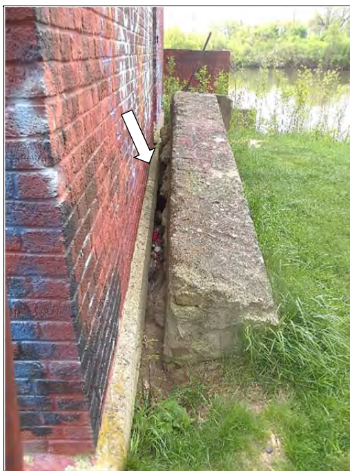
Photograph 3 – Large concrete barrier near the upstream wall of the powerhouse Note the large void under the barrier
