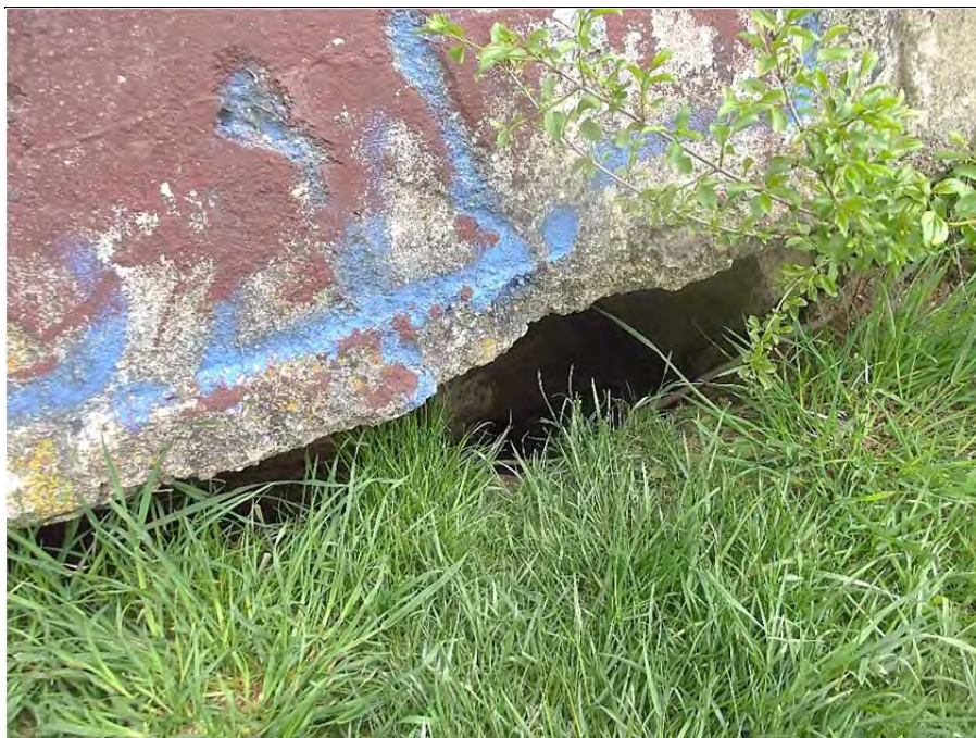
Photograph 4 – Close-up of the void under the barrier.
