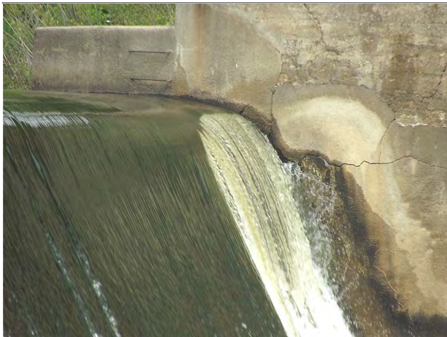
Photograph 14 – Deteriorated section of the principal spillway viewed from the right
