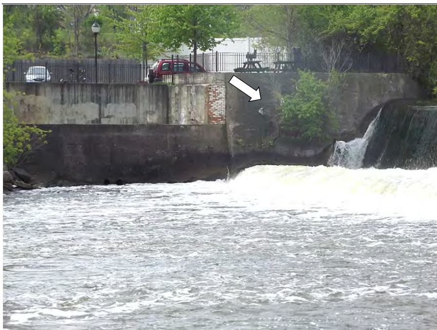
Photograph 18 – Downstream right principal spillway abutment wall Note the delamination and vegetative growth
