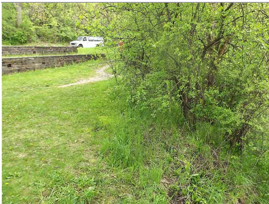
Photograph 6 – Downstream face of the left embankment viewed from the right Note the trees and brush
