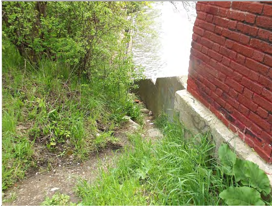
Photograph 7 – Foot traffic erosion at the downstream face of the left embankment
