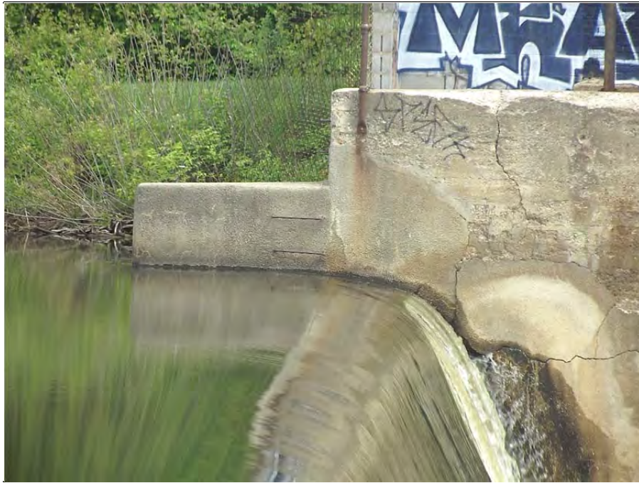
Photograph 15 – Upstream right principal spillway abutment wall Note the minor cracking and deterioration
