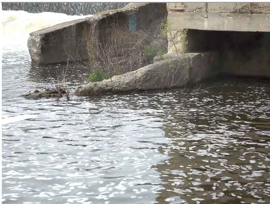
Photograph 24 – Close-up of the deteriorated training wall Note the vegetation
