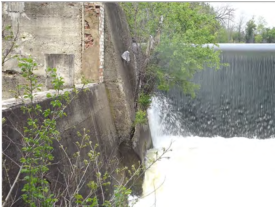
Photograph 20 – Delamination and vegetation viewed from downstream
