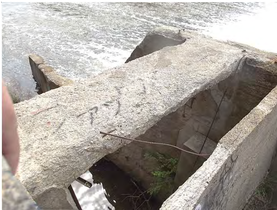
Photograph 22 – Auxiliary spillway outlet viewed from the left Note the deteriorated concrete and exposed reinforcing steel
