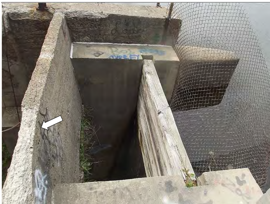
Photograph 21 – Auxiliary spillway viewed from the left Note the deteriorated concrete
