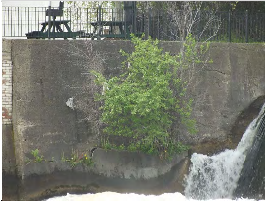
Photograph 19 – Close up of delamination and vegetation
